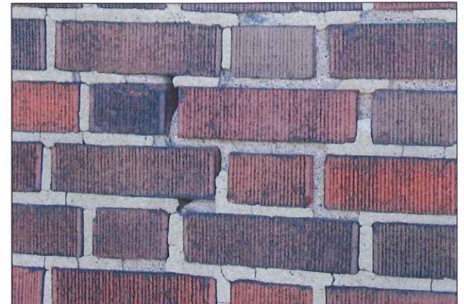
Previous poor repointing. Repointing mortar is falling out of joint due to improper execution.
