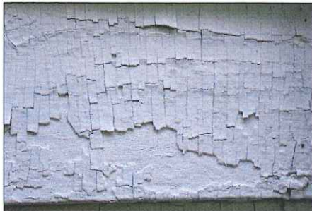
Alligatoring paint on exterior siding
