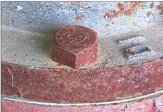
Galvanic corrosion resulting from a reaction between two dissimilar metals
