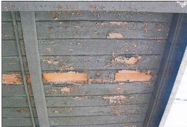
Paint failure on the underside of a wood canopy
