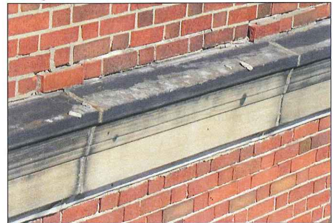
A loose stone cornice attached by metal fasteners indicate that its fasteners have failed.
