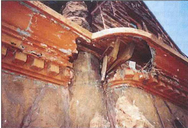
A painted lead-coated copper cornice is missing elements due to advanced deterioration of metal.
