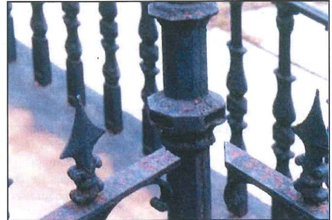
A corroded metal fence has failed at connections between the railings and the post.
