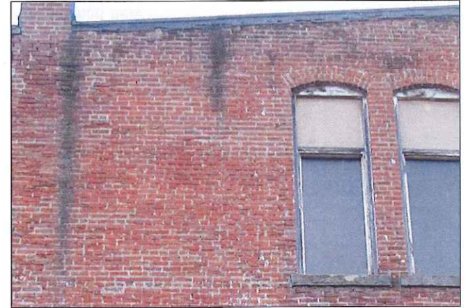
Dirt and stains on brick caused by runoff from the roof and corroded metal coping
