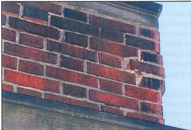
Displacement of brick caused by movement in the parapet wall
