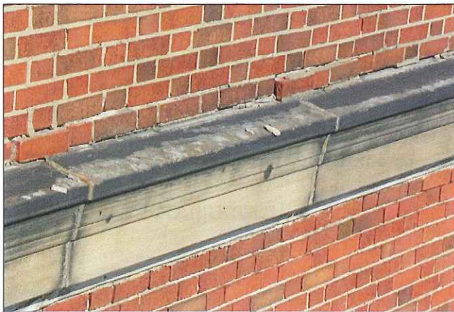
Loose brick falling out of wall due to poor condition of mortar joints
