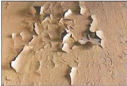
Peeling paint on interior wall
