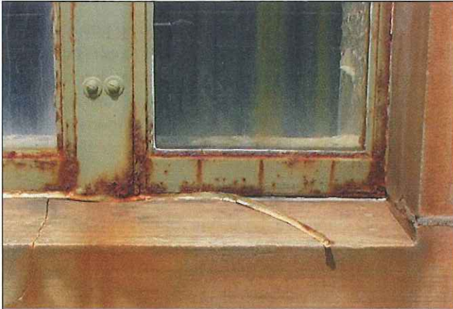
Corrosion/rust on a metal window sash resulting from exposure to moisture and air
